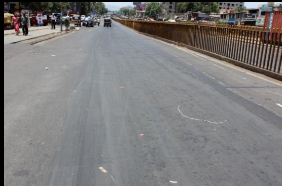
Next day of SEALKOTE application, visible surface undulations where asphalt has degraded on the right half of the asphalt road next to the concrete part
