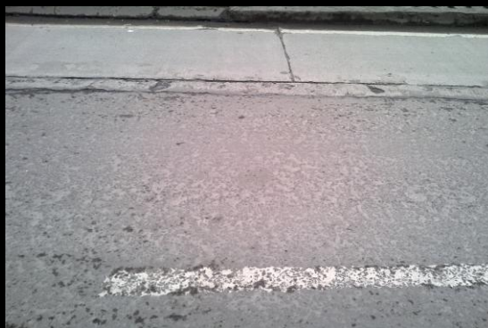
Surface as on 1 st August 2014, same condition as on the date of application after two seasonal rains no further damage, the gravel is still intact and SEALKOTE has held it together
