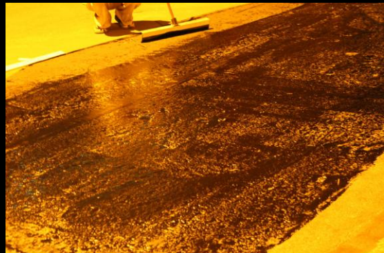
SEALKOTE application complete most of the coating has been absorbed by the porous and worn out surface
