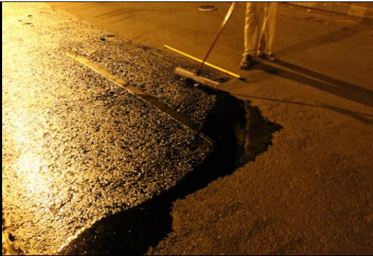
SEALKOTE application on most deteriorated surface at the rate of 1 Kg per SqMt done on 3 rd May 2012
