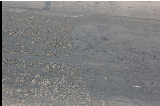
As can be seen the uncoated surface on the left has almost lost all binding of asphalt
