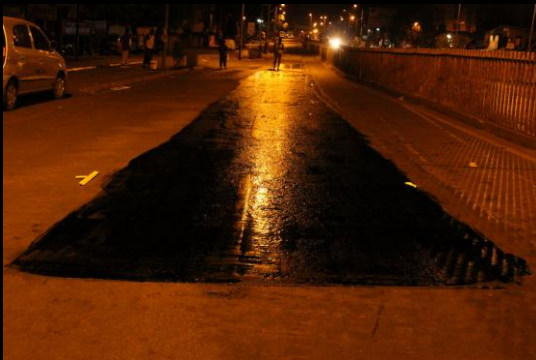
Application of SEALKOTE done on 150 SqMts of deteriorated surface having maximum traffic movement and maximum wear and tear
