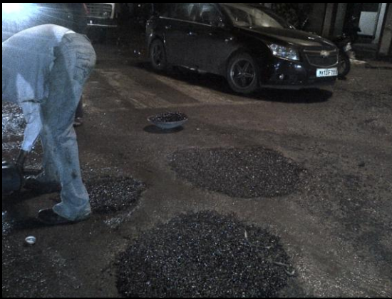
Next potholes filled with DBM (hot mix) into the SEALKOTE PATCH primed potholes
