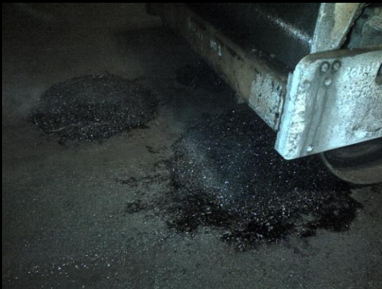
The repaired patch is compacted with a road roller and open to traffic immediately
