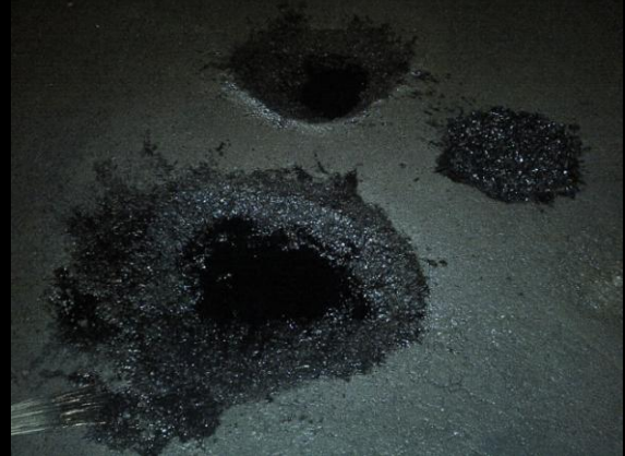
SEALKOTE PATCH applied as tack coat, visible penetration even in dirt filled pothole
