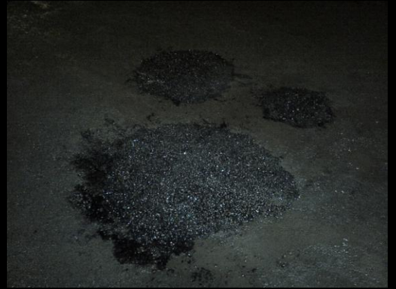
Fill pothole with an excess of DBM and have it suitably crowned and ready for compaction
