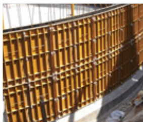
Interim Tank, ONGC, Mumbai, India
