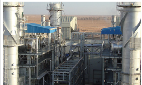
Thermax Boiler Plant, Algeria
