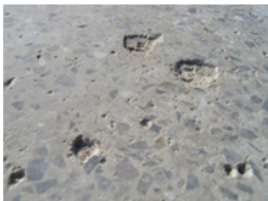
Pop outs in concrete
